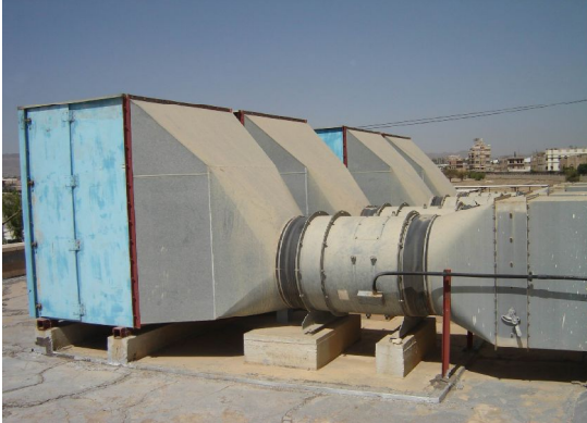
Air Filtration Unit for 2 MW Gas Engine in Yemen For Power plant ventilation & Engine filtration
