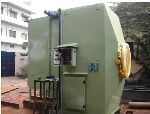
Air Intake System for Powerica DG set
